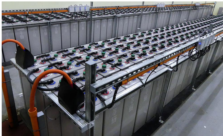
Fig 18.7: Industrial-Scale Battery Bank Installation for Large-Capacity Energy Storage Systems
