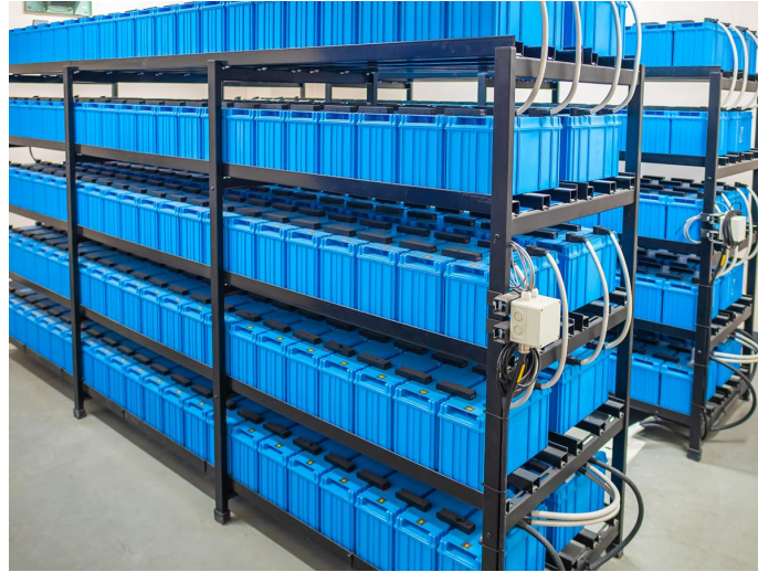
Fig 18.15: Modular Lithium-Ion Battery Rack System for Large-Scale Energy Storage Applications
